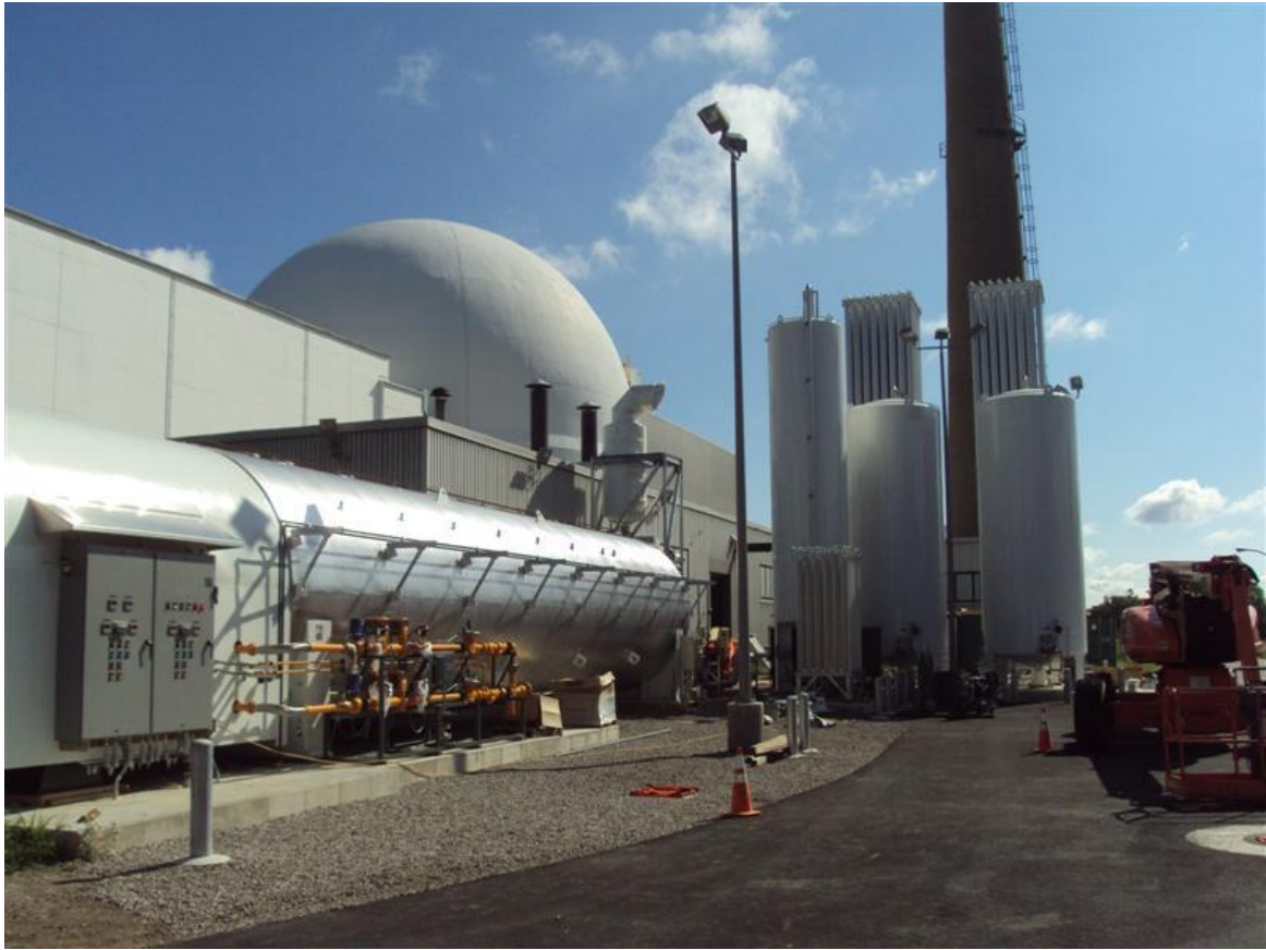
Figure 9: Construction photo showing the RATF nitrogen generation system, including the water-bath vaporizer and the liquid nitrogen tanks and vaporizers
