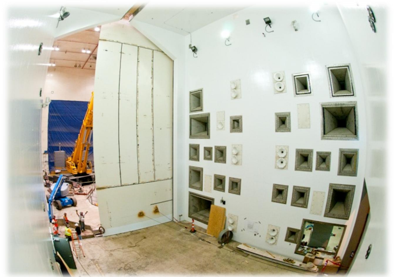
Figure 8: Construction photo with view of the RATF chamber and horn wall taken during the installation of the main sliding door
